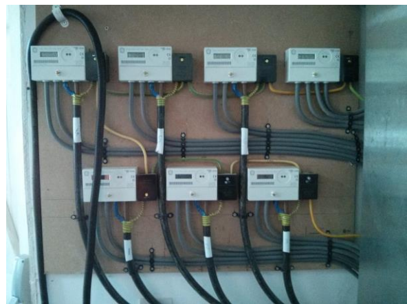
Figure 4 Soillse boiler room incomers in the Findhorn Community
